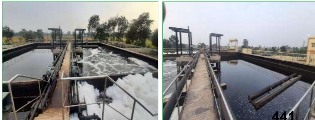
Rajnadgaon (Mohad): 6.2 MLD
